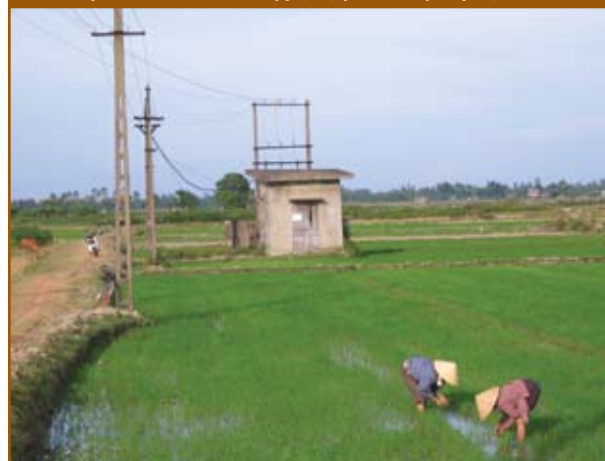
Example of a substation supplying power to pumping stations
