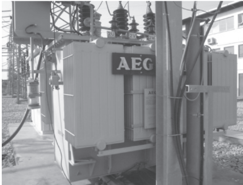
Picture A 9.4: Interposing Transformer at Techiman Substation
