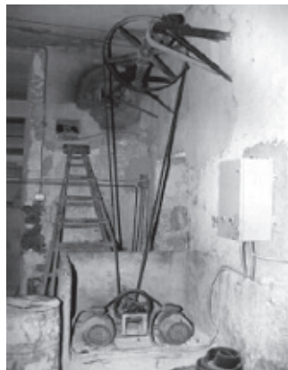
Picture A 1.8: Two Parallel Single-phase Motors Providing Additional Power for this Tunisian Industrial Client (Olive Oil Plant) (Cecelski, 2004)
