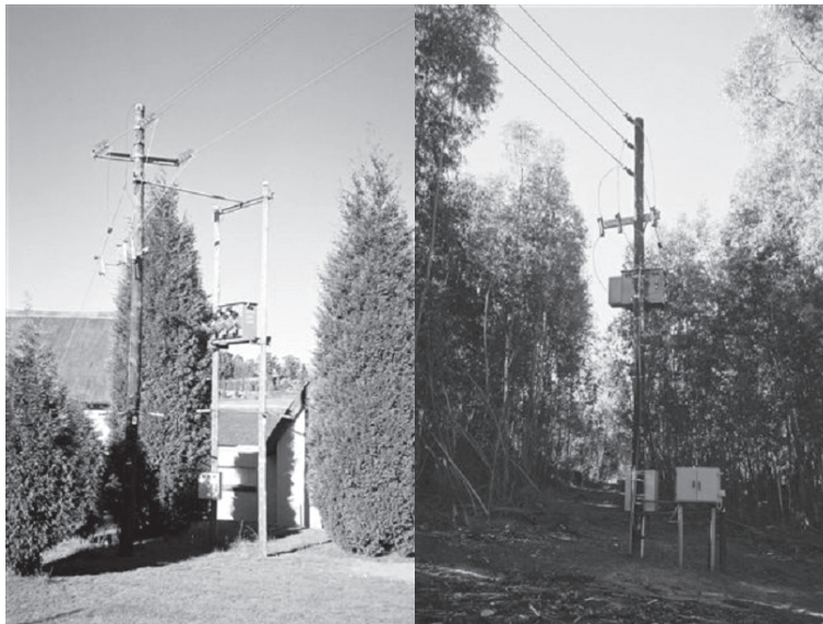
Picture A 2.2: The transformer on the left is 50 kVA and the one on the right 100 kVA
