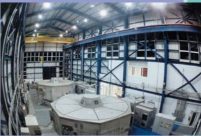
Inside powerhouse of the El Canada hydropower plant.
