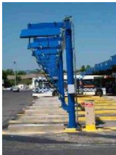
Figure 7: “Low refueling” CNG stations (Montpellier depot)
