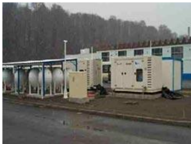
Figure 8: Details of the compression units and CNG tanks
