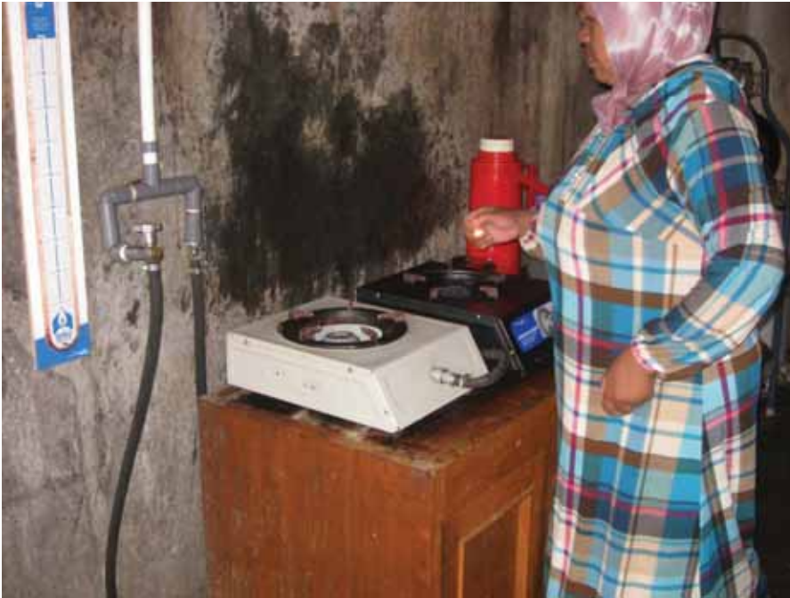
Gas Meter Level, Gas Pipe, Valve, and Stove in the Kitchen
