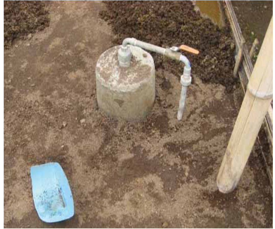
Gas outlet Valve and Gas Pipe from the Bio-digester is Piped to the Kitchen
