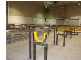
TUBE OUTFEED/INSPECTION/ BUNDLING
