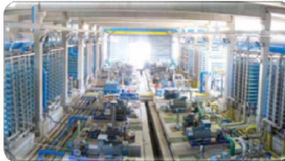
100,000 m³/day desalination plant (India)
