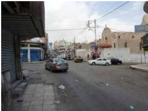
Poor Quality Footway
