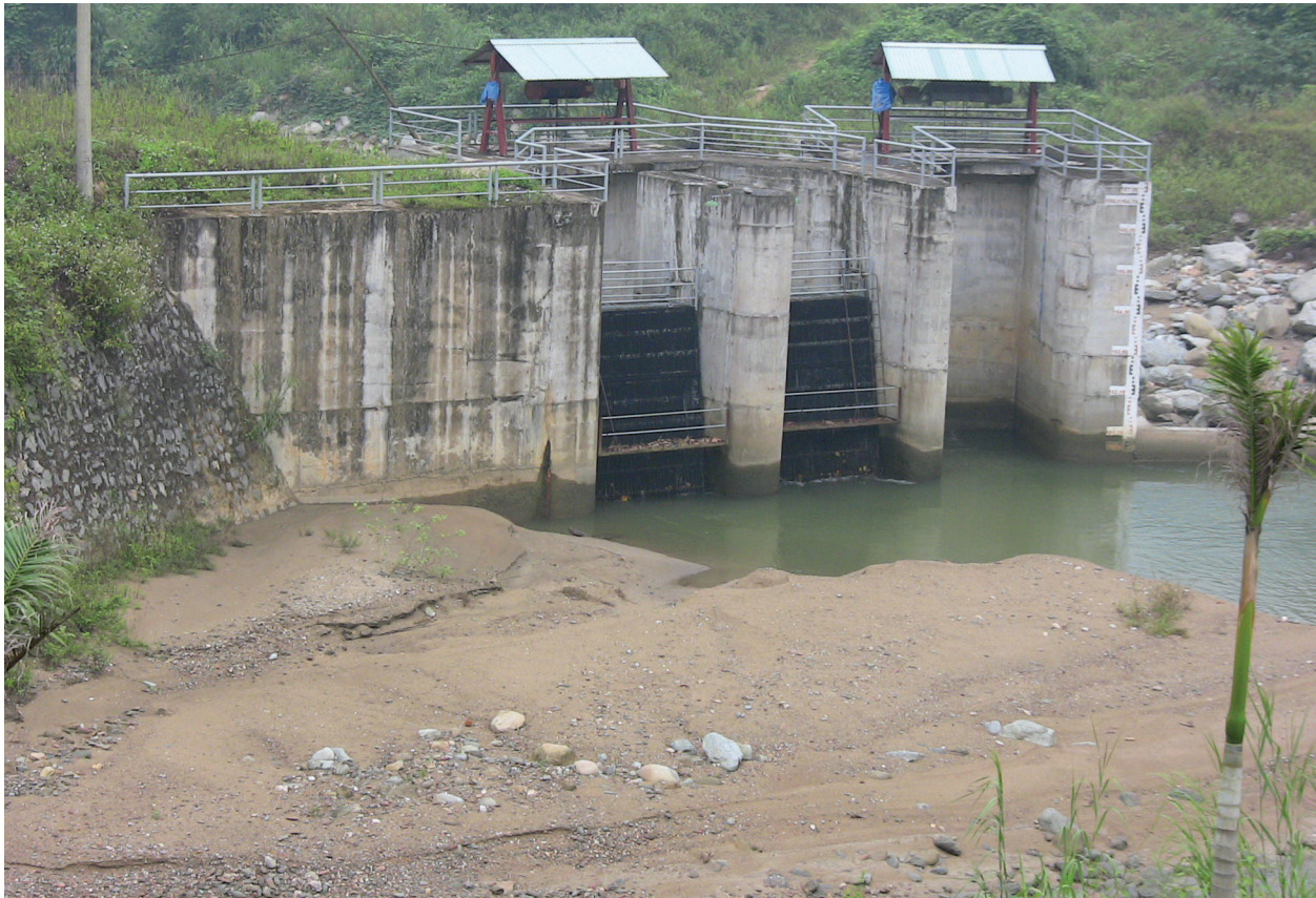
PHOTO 6.1 SEDIMENTATION IN FRONT OF THE INTAKE OF VAN HO SMALL-SCALE HYDROPOWER PLANT IN THE NGOI XAN BASIN (LOOKING DOWNSTREAM)
