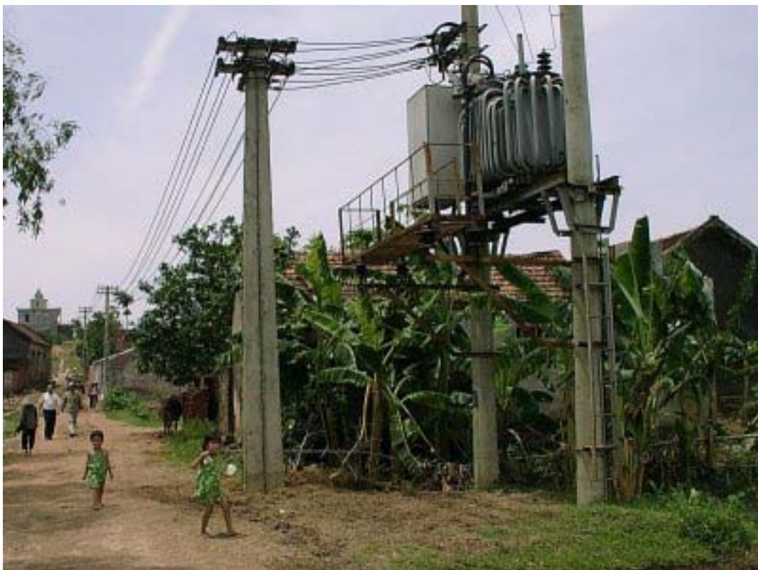
Figure 1-3: Substation in Hoi Phu where the load was metered
