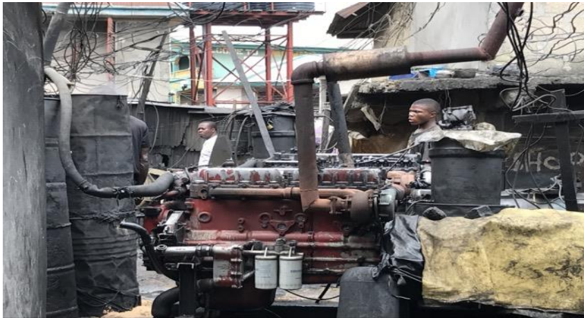
One of the general generators used within the Market
