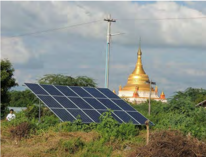
One of three identical 3.6 kW solar powered mini-grids that power Myin Chi Naing village. Photo by Eric Youngen
