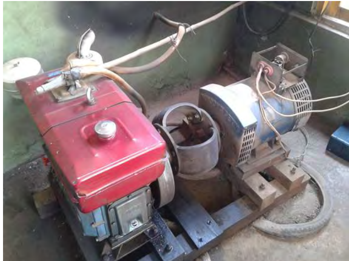
Diesel generator at Ton Lon village. Photo by Chris Greacen
